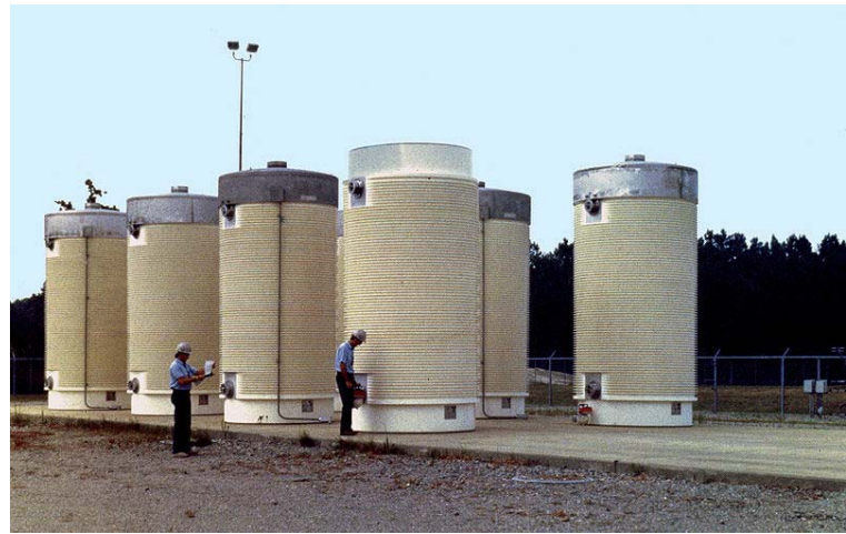
Dry Storage Facilities
